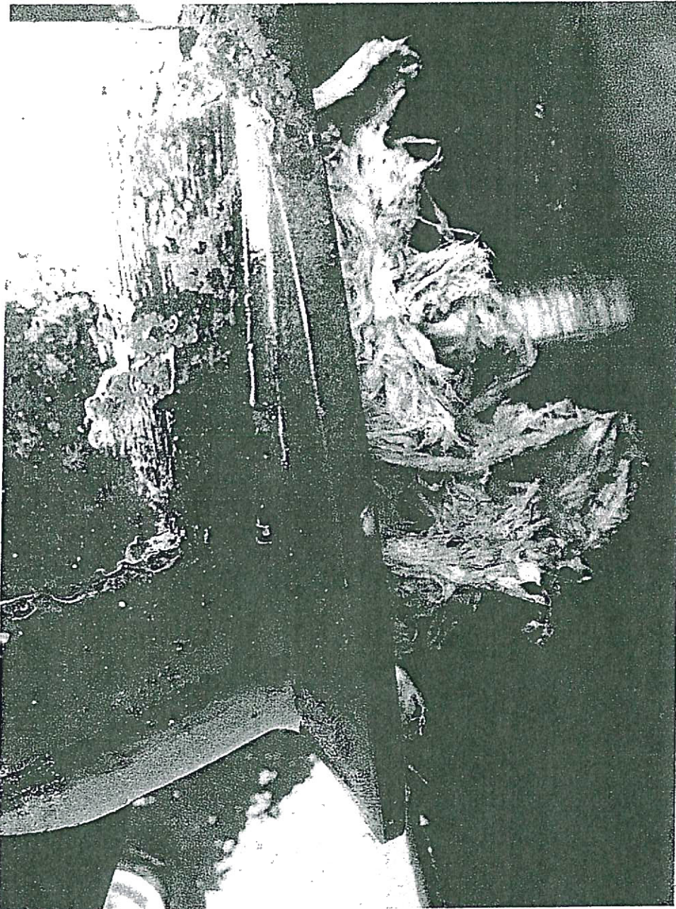
The influent pump at our Waste Water Treatment Plant developed this rag ball one week after being rebuilt. The pump has already failed. (Photo May 2019)
